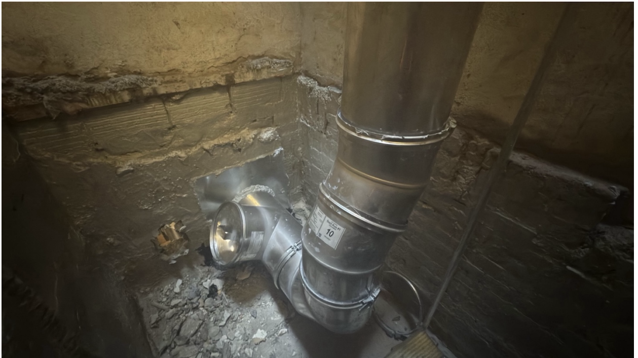
Photo Credit: Master Fire 4 The duct system carries contaminated air from the hood to the outside of the building.
