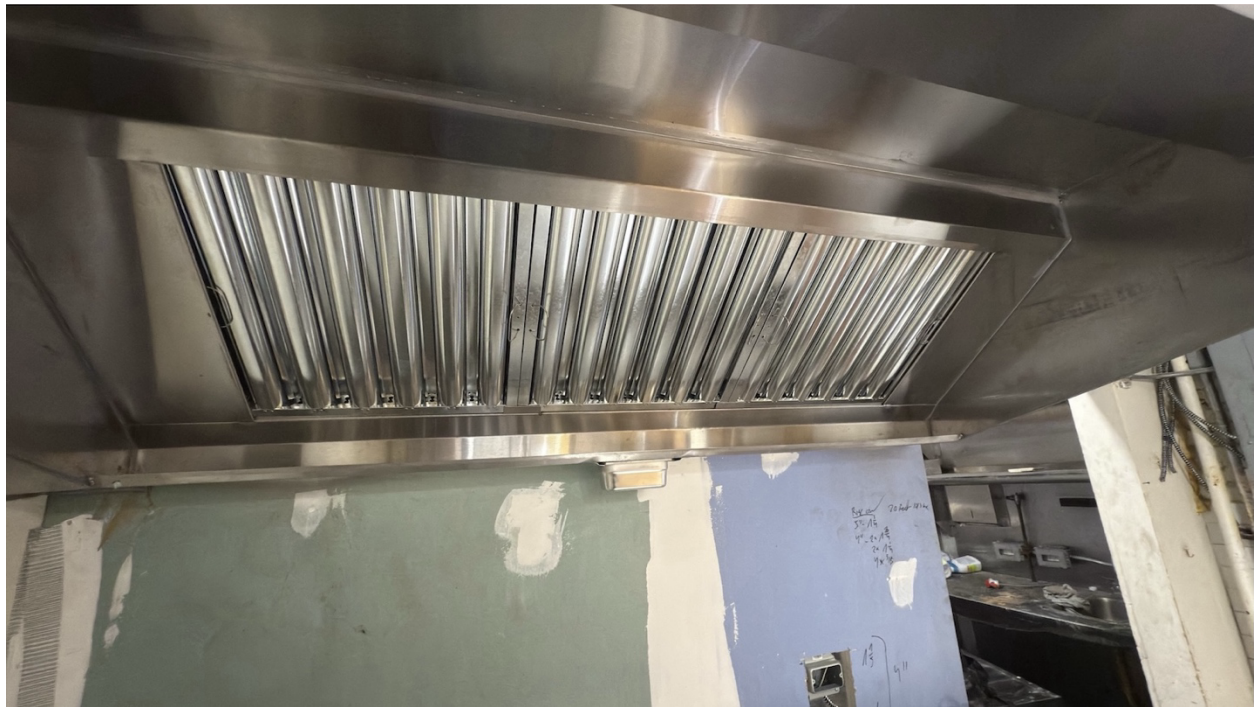
Photo Credit: Master Fire 1 The removable grease cup collects runoff and reduces the fire hazard inside the ductwork.
