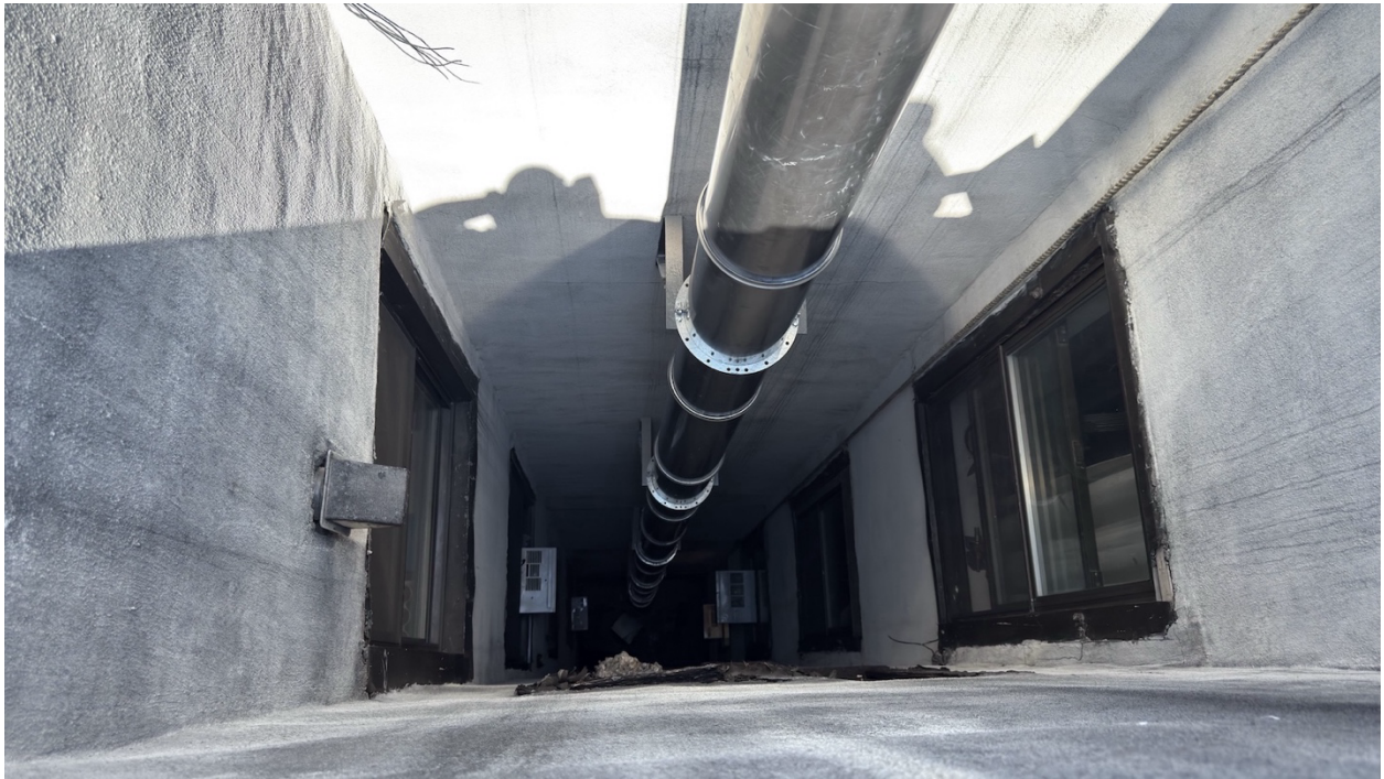
Photo Credit: Master Fire 5 Precision-fabricated ducts ensure airtight seams and smooth airflow.
